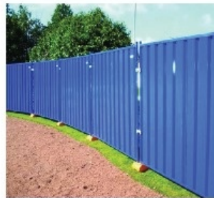
Running Hoarding Fence
